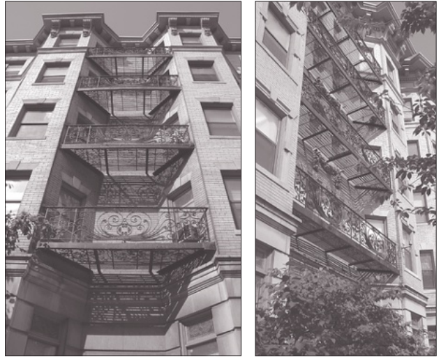
The wrought iron grill work between some windows are considered fire escapes and are for emergencies only.
