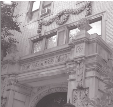
The “wells” above the entrances are NOT balconies.
