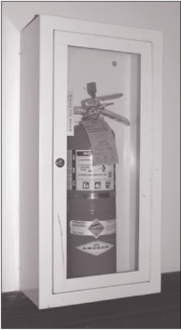
Fire extinguishers are located near the elevators
